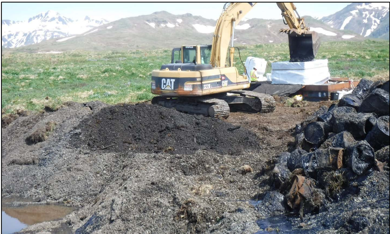
Figure 2. Photograph taken June 2016 showing an excavator loading drum carcasses, leaked asphalt, and contaminated soil into a polymer shipping bag.
