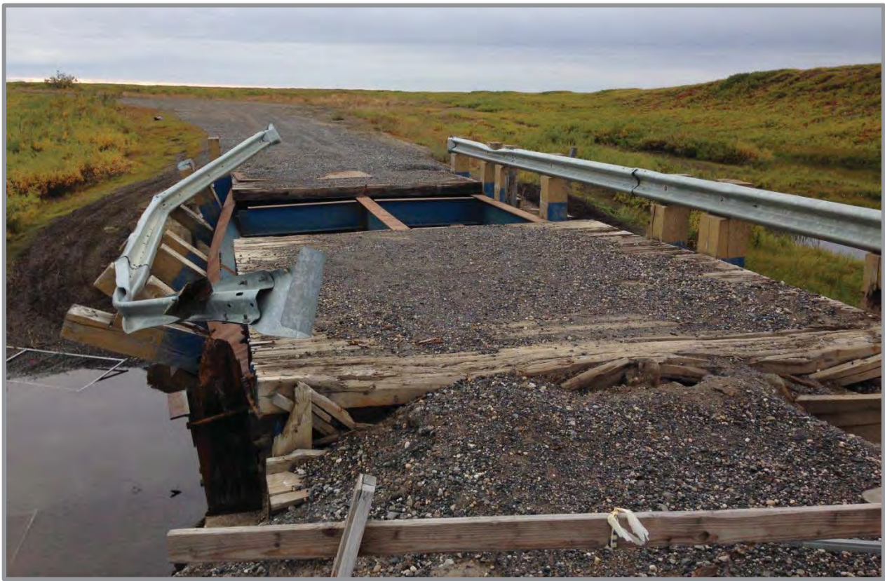
Figure 4: Failed Bridge at Site 2
