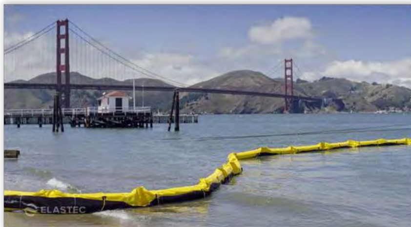
Figure 5-31. Type III Ruffwater Screen Turbidity Curtain being deployed in San Francisco Bay, CA.
