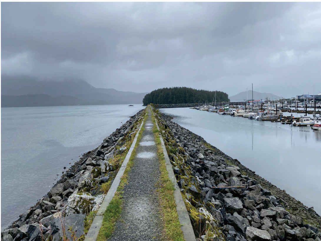
Condition of the western breakwater, August 2020.
