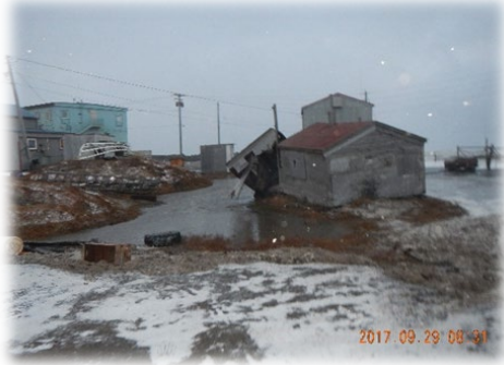
Barrow Coastal Erosion DRSA $364M Total Cost: $364M
