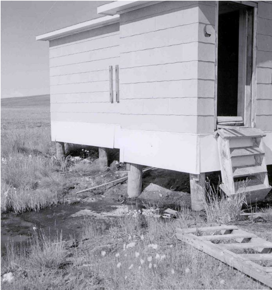
Umiat, Alaska, July 1958 Equipment building at MRL site. Foundation, siding and roofing in same condition as constructed. Floor is warped because of open door. Note thawed tundra in foreground caused by disturbing surface cover.
