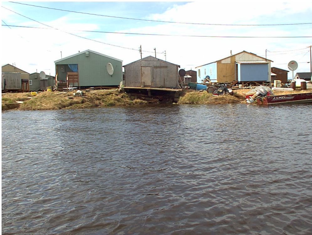
Photo 2: Land under house eroded out dated 16 June 2008
