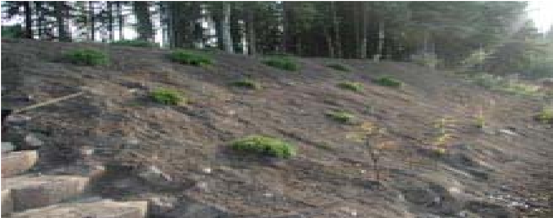
Photo 1: Bio-engineered restoration of rapidly eroding bank of the Chena River at River Bend Estates included placing a log berm at the toe with willow-staked riprap upslope, and planting birch and juniper trees at the top of the bank. Photo courtesy of the USFWS, No photo date.
