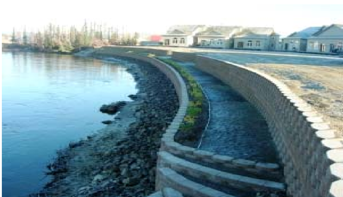
Photo 2: Summit Consulting engineered a 400-foot double tiered retaining wall along the north side of the Chena River to prevent erosion at the Riverbend Condominiums site at Doyon Estates; Photo courtesy of Summit Consulting Services, Inc. 2005.
