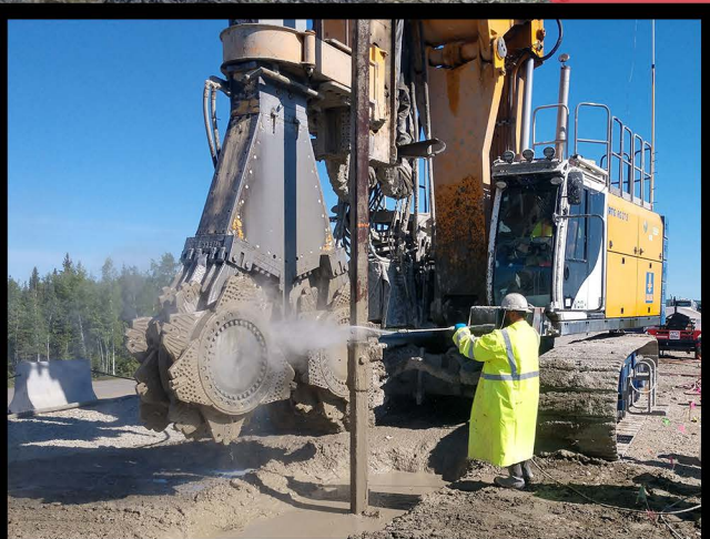
Work involves constructing 4.5 miles of mix-in-place concrete barrier wall to depths of up to 65 feet
