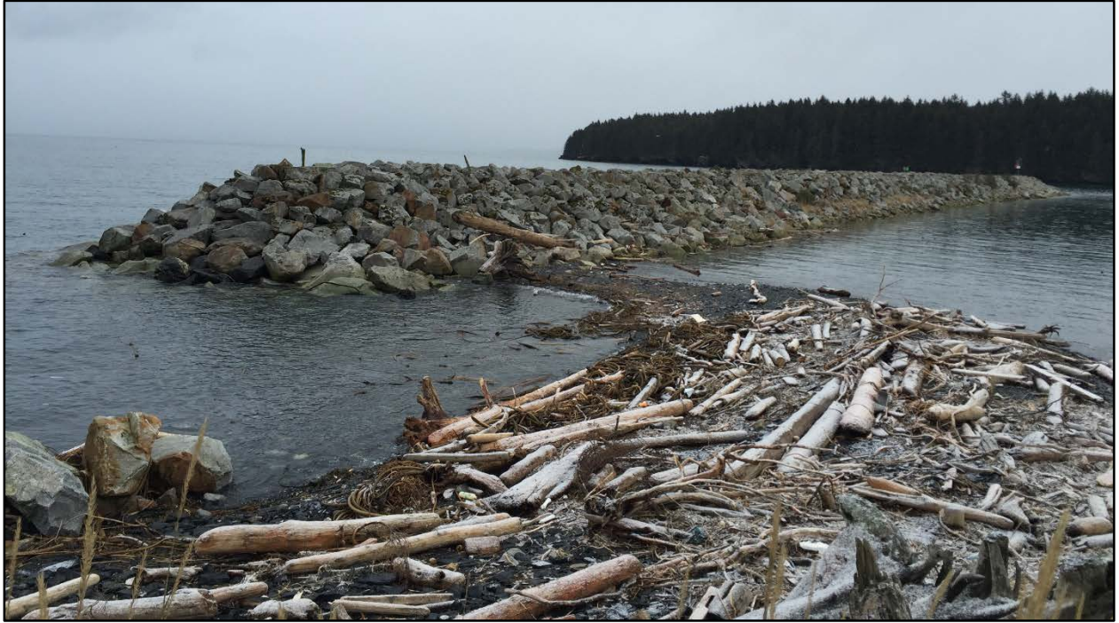
Figure 2. A 4 March 2016 view of the west end of the existing main breakwater and the fish passage gap, during a high tide of 8.5 feet above MLLW; note that fish passage is blocked by sediment even during this high tide, and the accumulation of large woody debris that has been driven into the gap.
