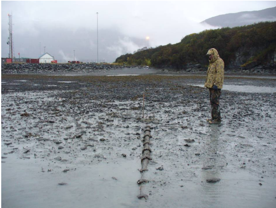
Photograph 6: Partially buried primary fiber optic cable.
