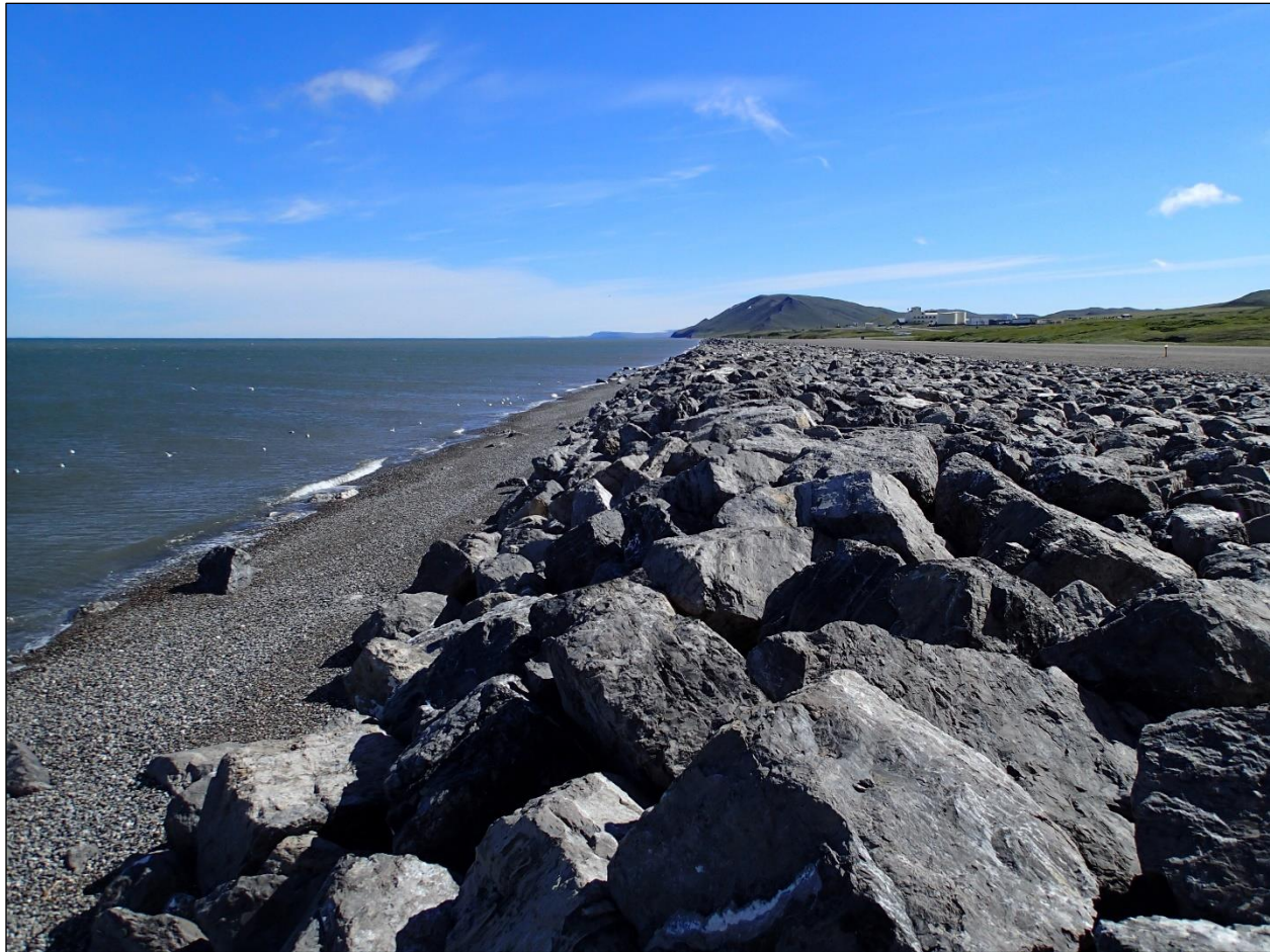
Figure 7. An example of a rock revetment from a USACE project on Cape Lisburne (about 280 miles SW of Barrow). Armor rocks shown are approximately 3.5 tons each.
