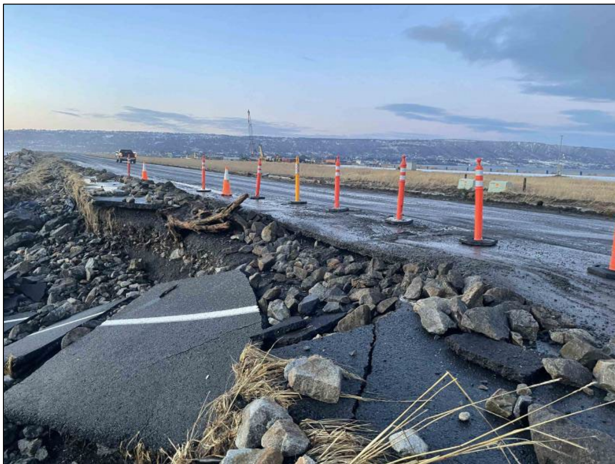
Figure 3-18. Highway partially collapsed after 2024 Storm Surge
