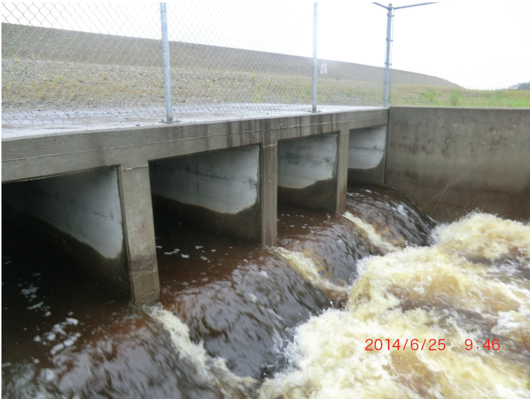
Downstream portion of the Low Point Drain during the 2014 flood event
