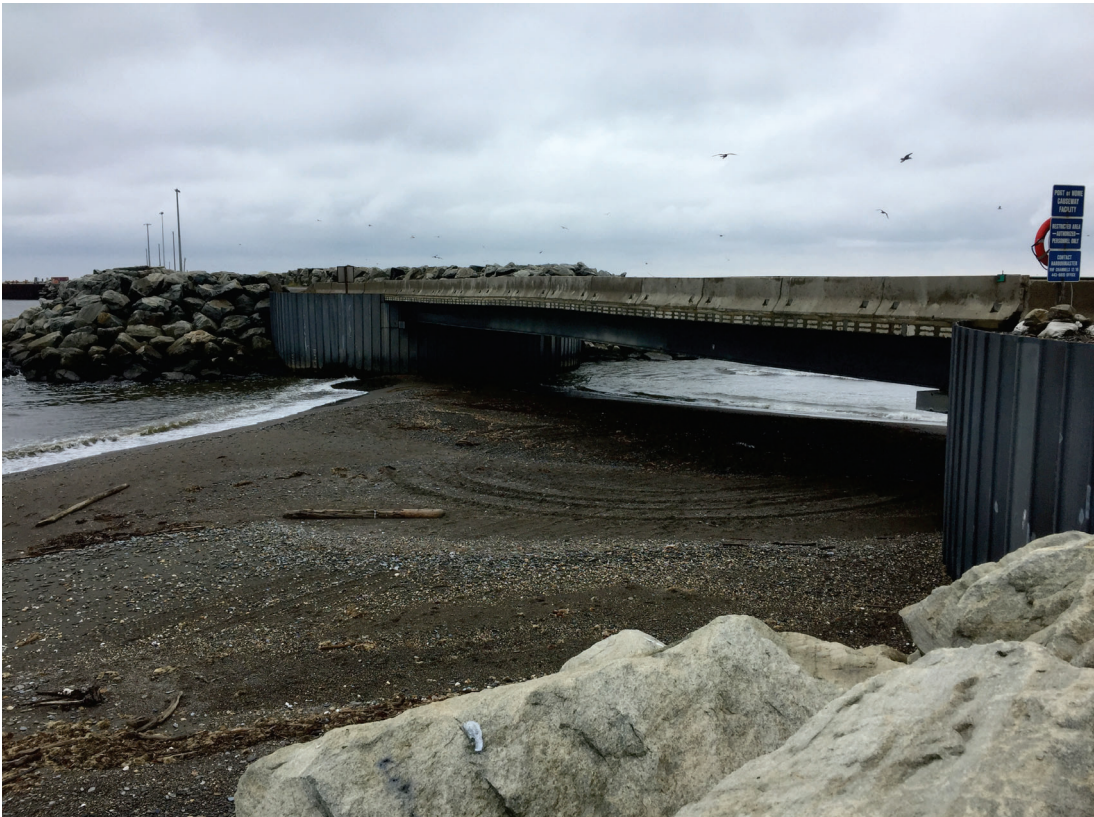
Significant shoaling under the causeway bridge, September 2018
