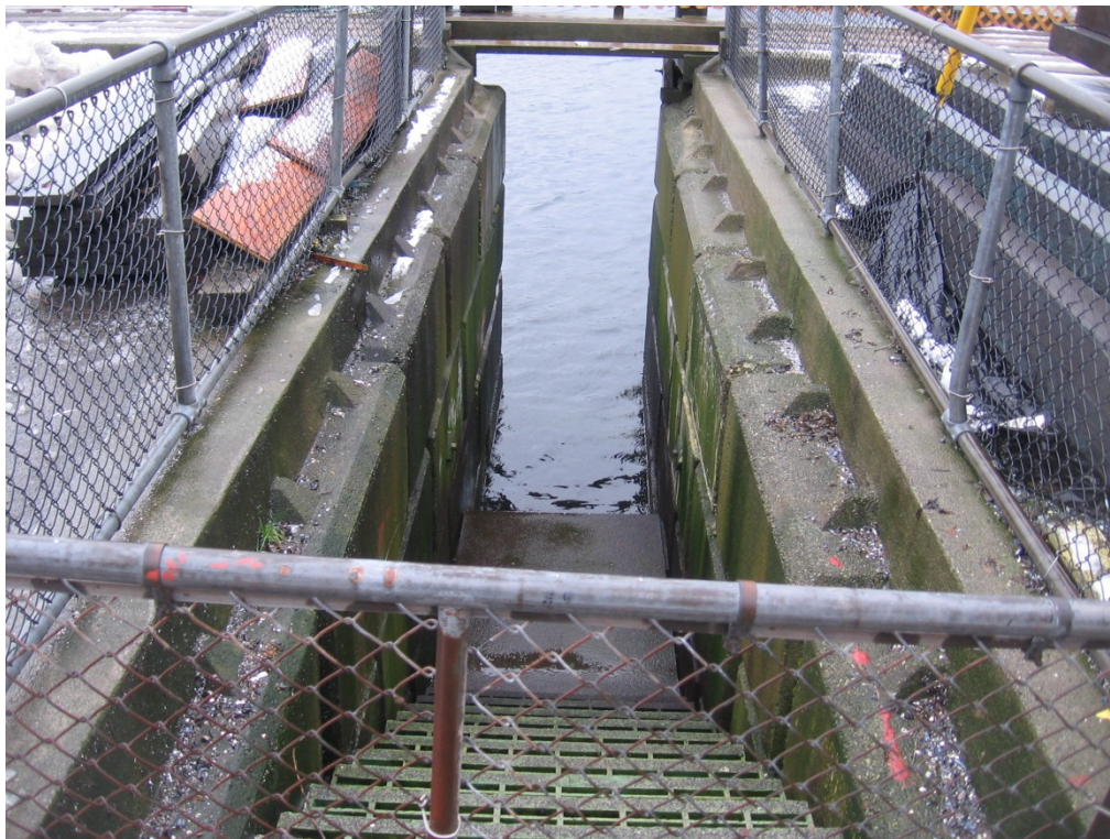
Figure 6 - Existing failing retaining wall and staircase
