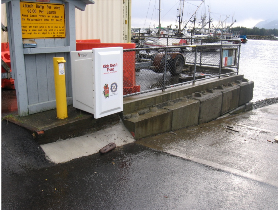
Figure 5 - Failing Retaining Wall and Concrete Abutment
